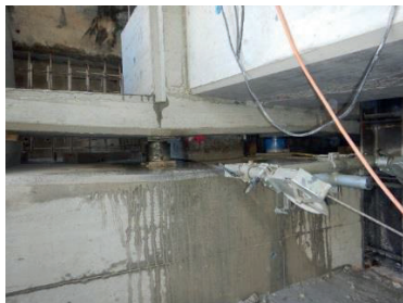
Figure 13. Bridge deck resting on the new concrete supporting bloc during the jacking
